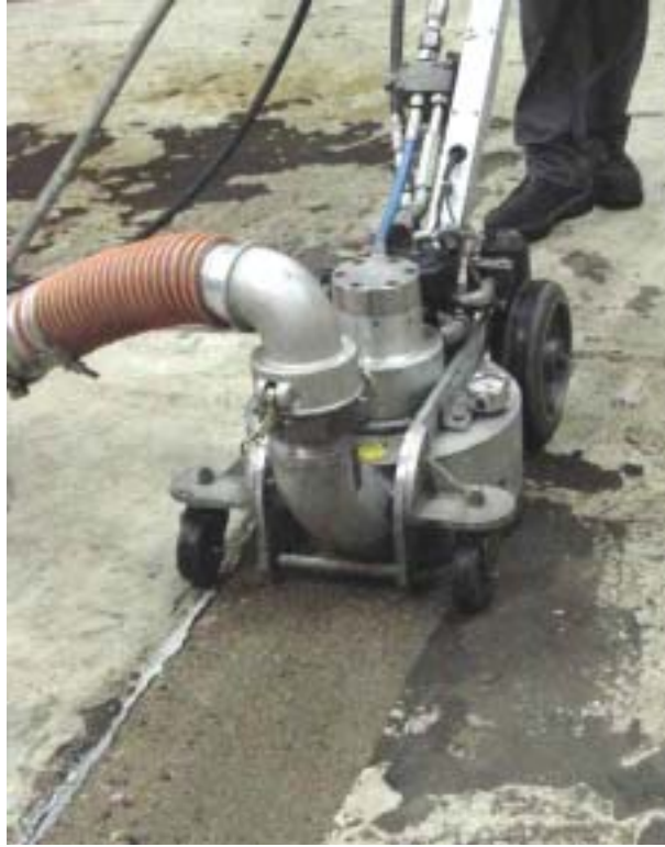
Figure 3. Semi-automated tools are the most popular for performing coating removal from concrete.
